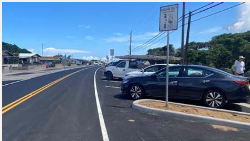
The 'Onehe'e Complete Street Project includes roadway reconstruction, raised and protected bicycle lanes, back-in angled parking, new sidewalks and curb ramps, and landscaping.
